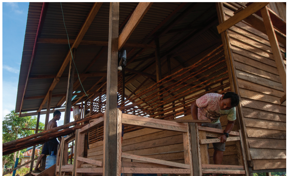
Construction of the Training Centre and gallery in Sungai Canggai © M. Aldi Khatami
